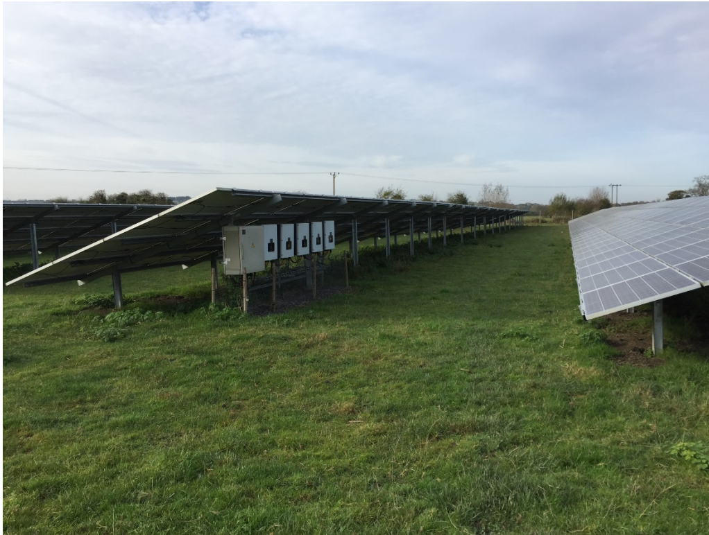
Plate 2 – Example image of string inverters mounted to Mounting Structures beneath the PV Modules
